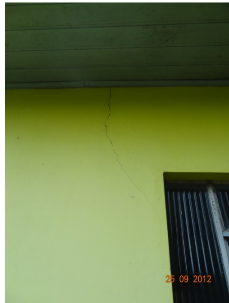
Fissura Janela Lateral (25/09/2012, 10:44h)
