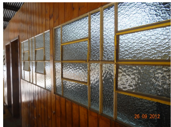
Forro Quarto (26/09/2012, 15:48h)
