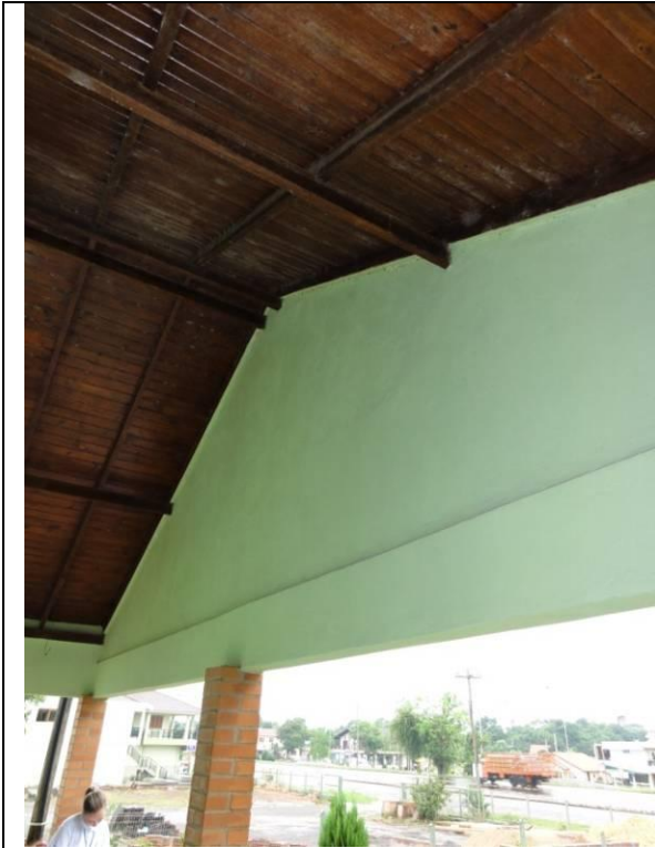
Fachada – Area - Teto (DSC04251, 23/02/2011, 17:16h)
