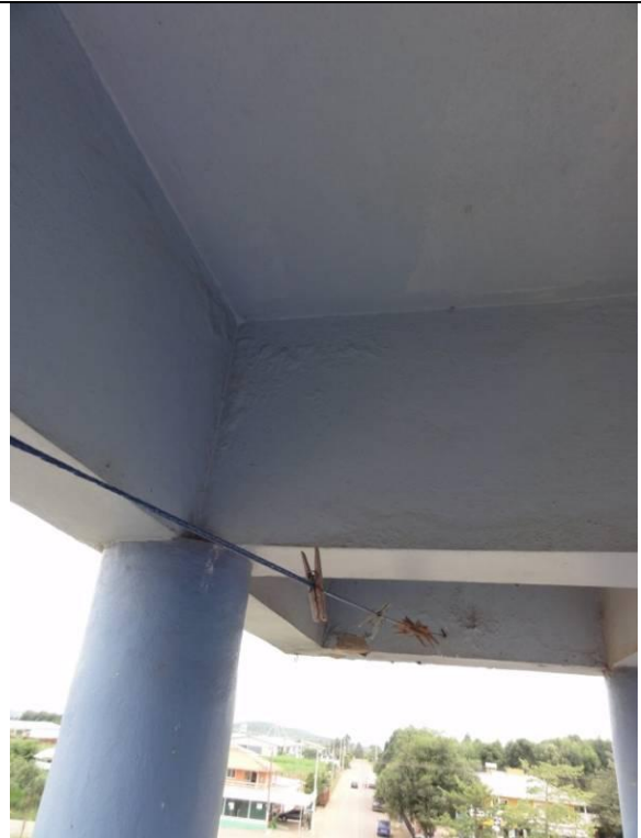
Piso superior –Sacada – Marquise (DSC02355, 21/02/2011, 16:09h)
