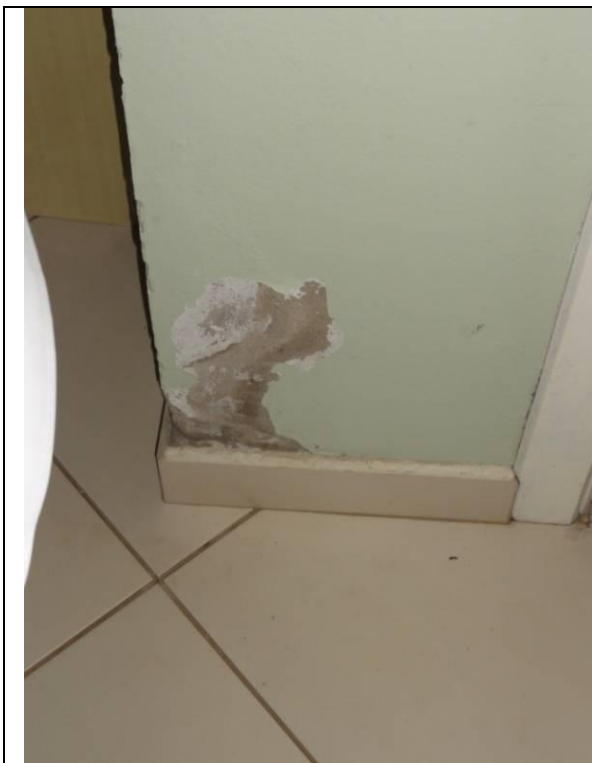
Piso superior – Quarto 3 – Reboco descascado (DSC03000, 22/02/2011, 10:25h)
