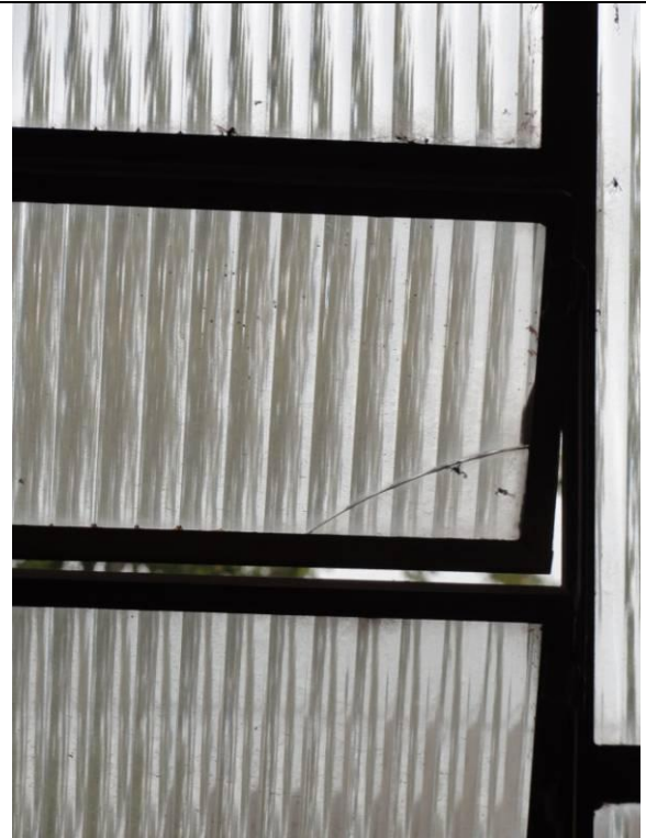
Piso inferior – WC – Janela rachado (DSC02828, 22/02/2011, 09:43h)
