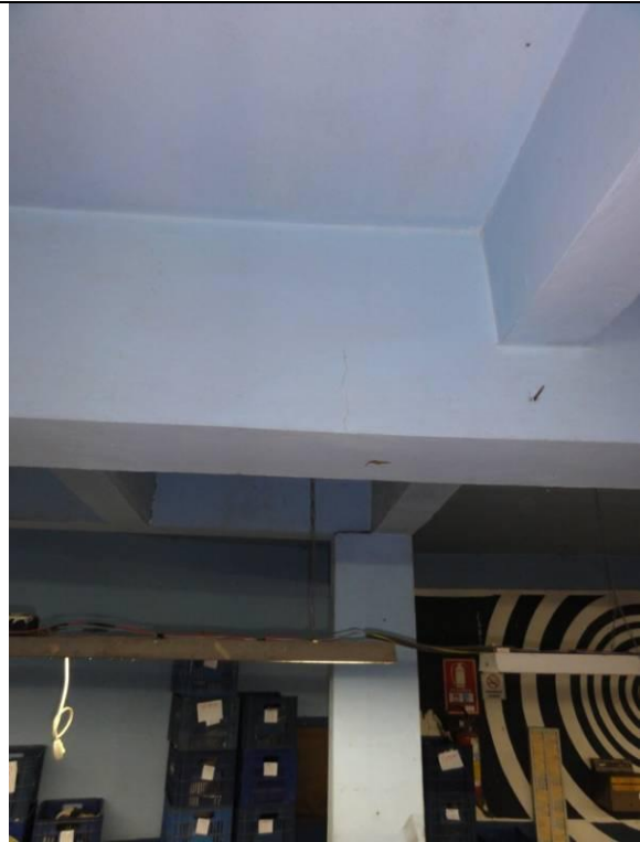
Piso Inferior – Fábrica – Teto (DSC03112, 22/02/2016, 11:28h)
