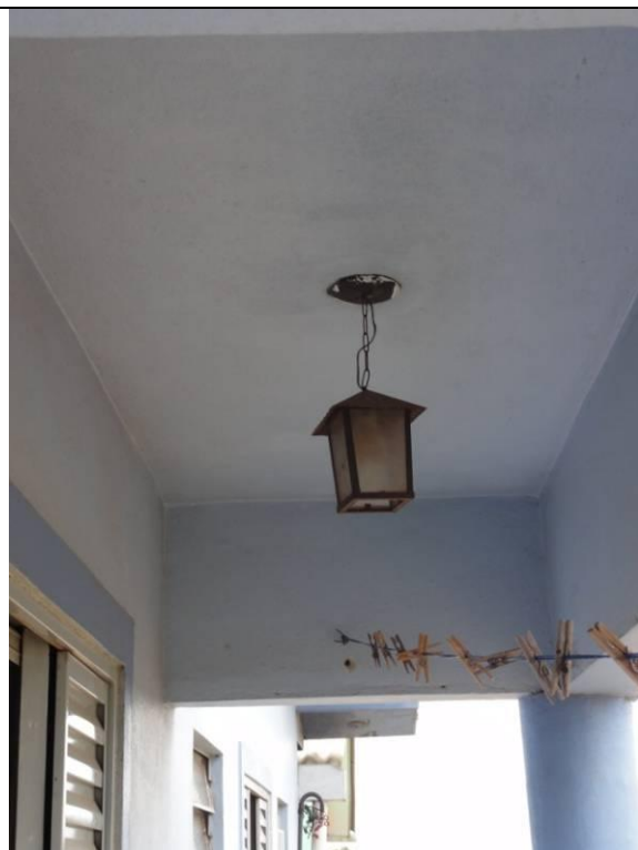
Piso superior – Sacada – Marquise (DSC02345, 21/02/2011, 16:08h)
