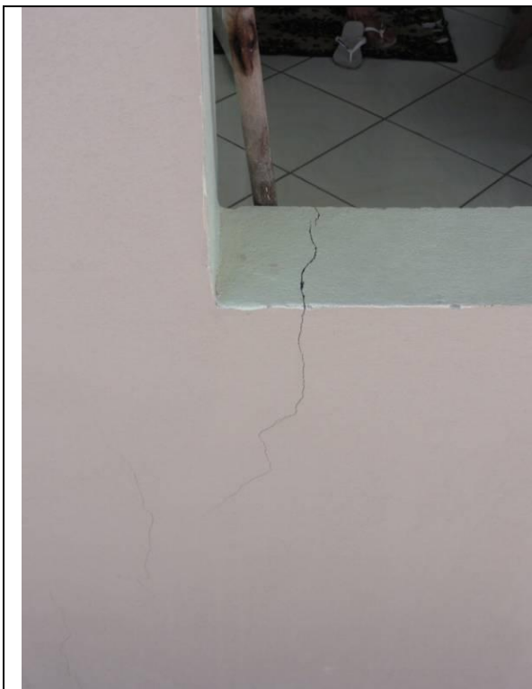
Piso superior - Fundos – Sacada – Fissura no reboco (DSC01042, 16/02/2011, 14:14h)
