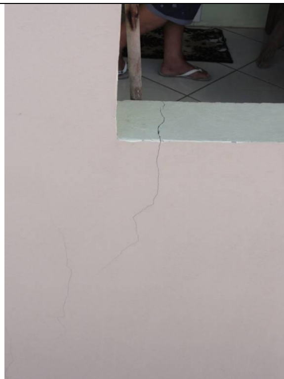
Piso superior - Fundos – Sacada – Fissura no reboco (DSC01041, 16/02/2011, 14:14h)
