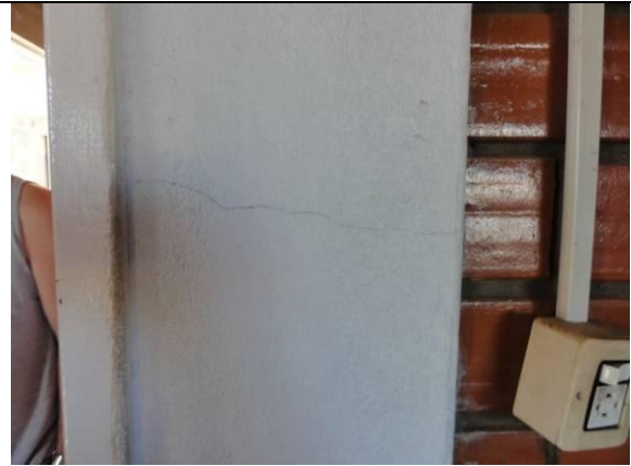
Apto 5 – Sala – Fissura no reboco (DSC00655, 16/02/2011, 09:28h)
