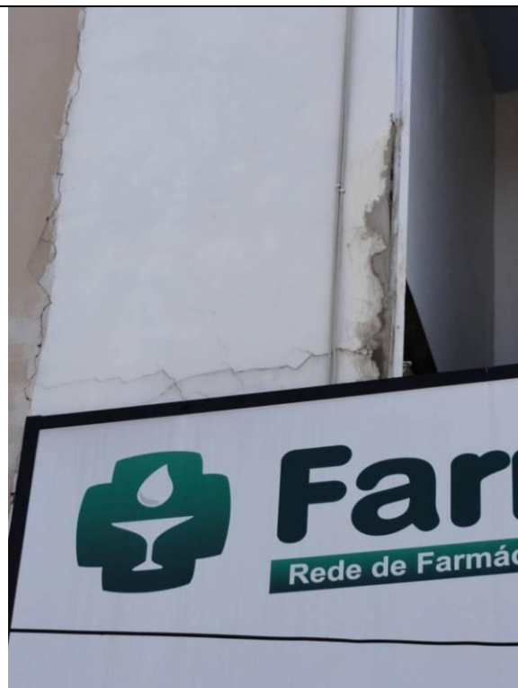
Fundos – Parede com rachadura no reboco (DSC01105, 17/02/2011, 07:20h)
