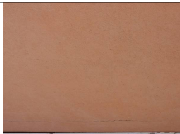
Piso superior – Sacada – Parede com fissura no reboco (DSC00677, 16/02/2011, 09:34h)
