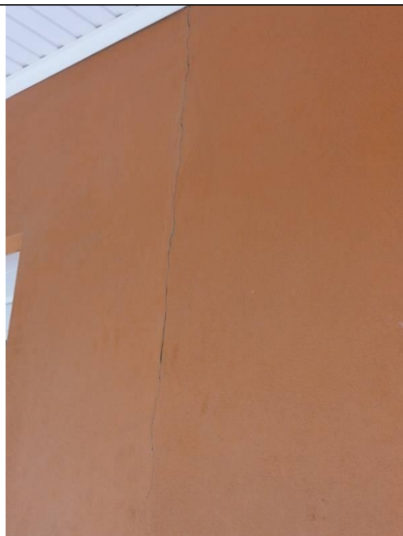
Piso superior – Sacada – Parede com fissura no reboco (DSC00675, 16/02/2011, 09:34h)
