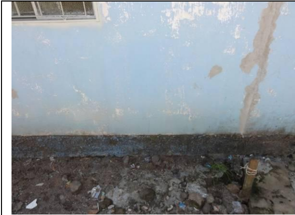
Lateral B - Reboco descascando (DSC01511, 17/02/2011, 10:45h)
