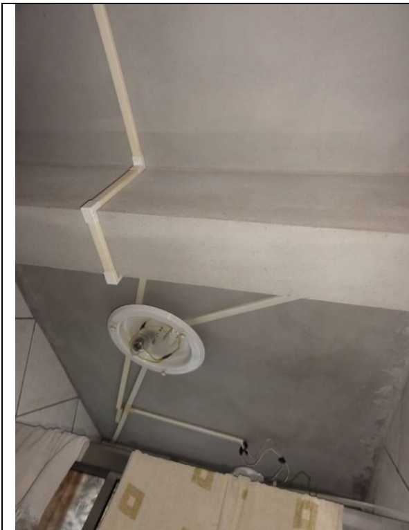
Apto 5 – WC - Teto (DSC00660, 16/02/2011, 09:30h)
