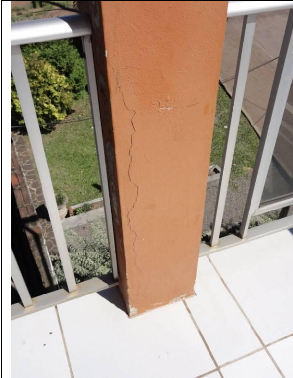
Piso superior – Sacada – Fissura no reboco (DSC00762, 16/02/2011, 10:00h)
