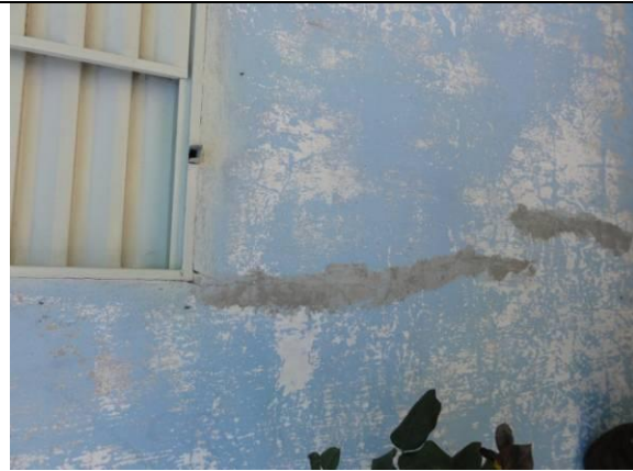
Lateral B - Reboco descascando (DSC01512, 17/02/2011, 10:45h)
