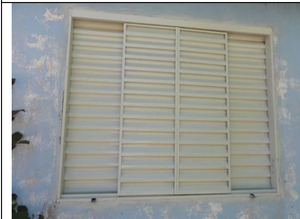
Lateral B - Reboco descascando (DSC01513, 17/02/2011, 10:45h)
