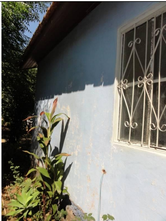
Lateral D - Janela (DSC01497, 17/02/2011, 10:42h)
