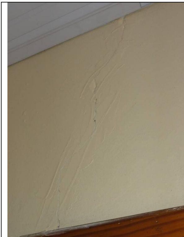
Sala – Fissura reboco (DSC00191, 15/02/2011, 14:06h)
