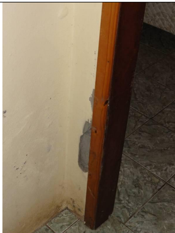
Reboco descascado (DSC00051, 15/02/2011, 13:34h)
