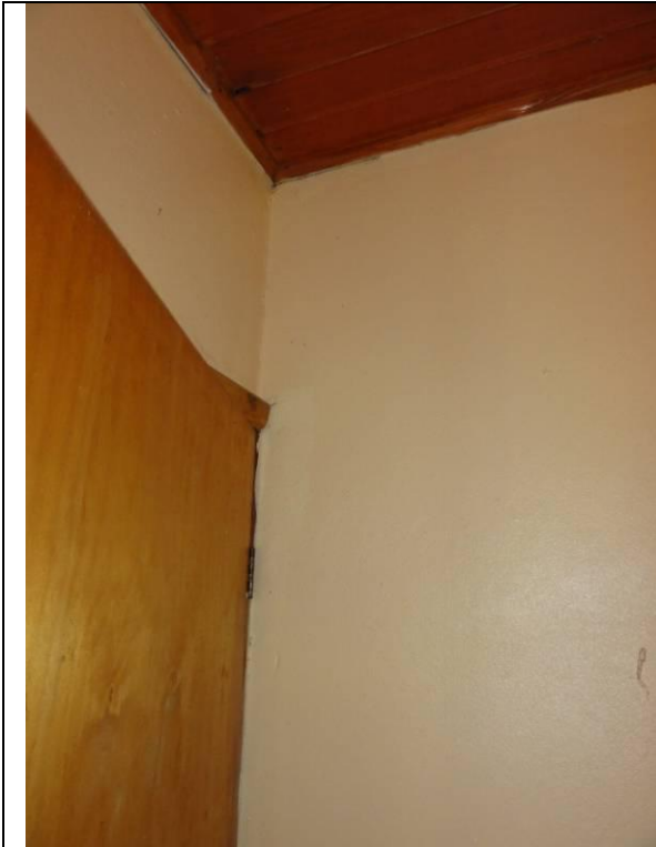
Fissura no reboco (DSC00066, 15/02/2011, 13:37h)
