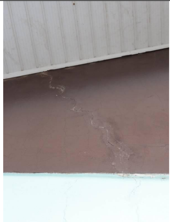
Fissura no reboco – Parede A(DSC00131, 15/02/2011, 13:54h)
