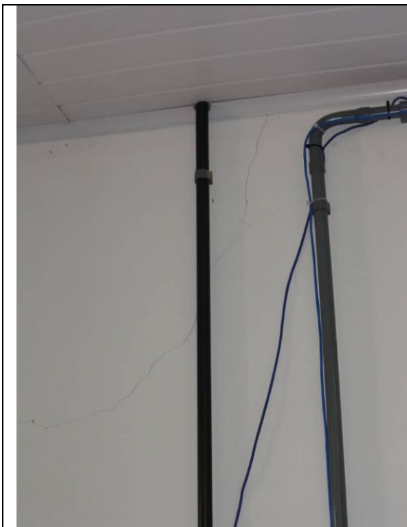
Sala 5 – fissura no reboco (DSC01916, 18/02/2011, 08:23h)
