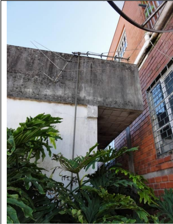
Fundos – Fissuras no reboco (DSC00539, 16/02/2011, 08:27h)
