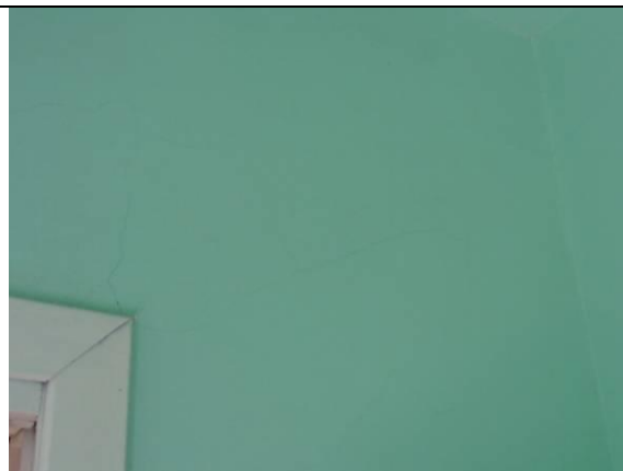
Apto 301 – Fissura no reboco (DSC02064, 18/02/2011, 09:05h)
