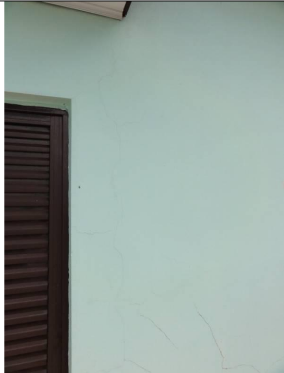
Leve fissura no reboco (DSC00101, 15/02/2011, 13:50h)
