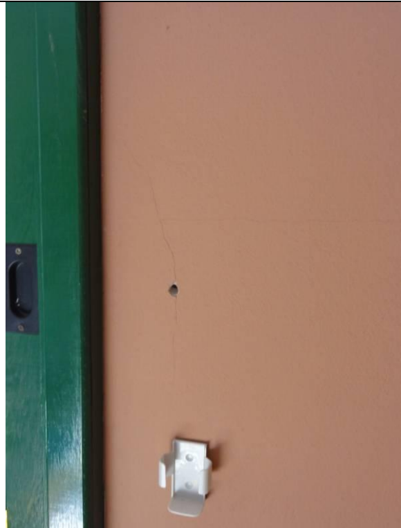
Sala 6 – Fissura no reboco (DSC01963, 18/02/2011, 08:35h)
