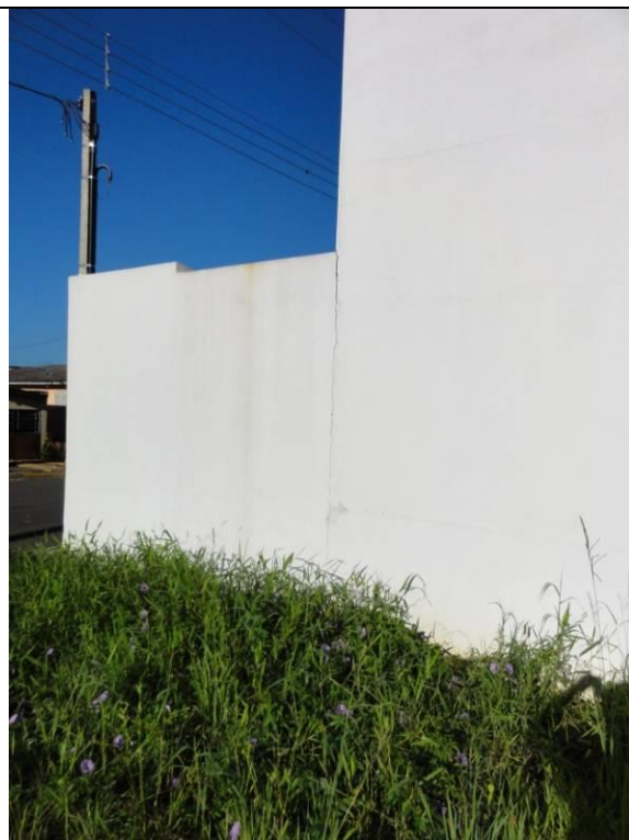
Lateral C – Fundos – Rachadura na parede (DSC00452, 16/02/2011, 07:54h)
