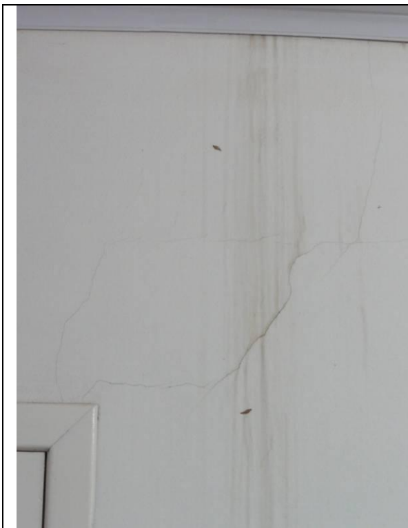
Sala 2 – Fissura no reboco (DSC01872, 18/02/2011, 08:07h)
