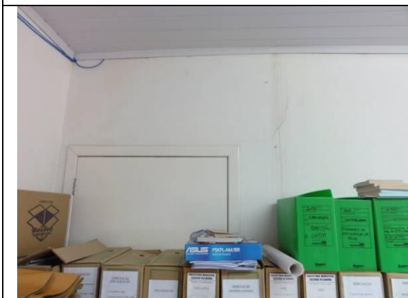
Sala 2 – Fissura no reboco (DSC01870, 18/02/2011, 08:07h)
