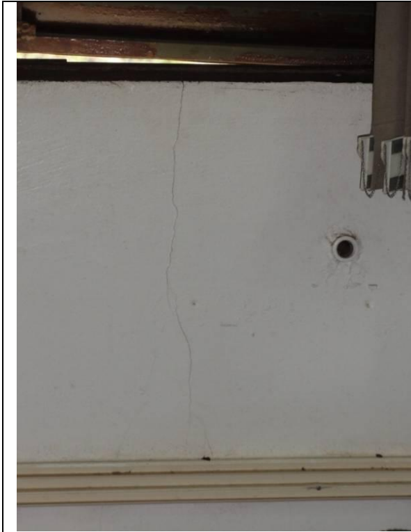
Fissura no reboco (DSC00569, 16/02/2011, 08:34h)
