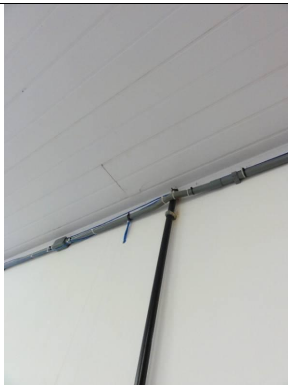
Sala 5 – fissura no reboco (DSC01919, 18/02/2011, 08:25h)
