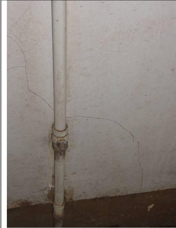
Lateral D – Fissuras no reboco (DSC00553, 16/02/2011, 08:30h
