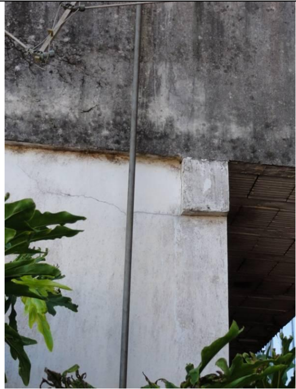
Fundos – Fissuras no reboco (DSC00540, 16/02/2011, 08:28h)
