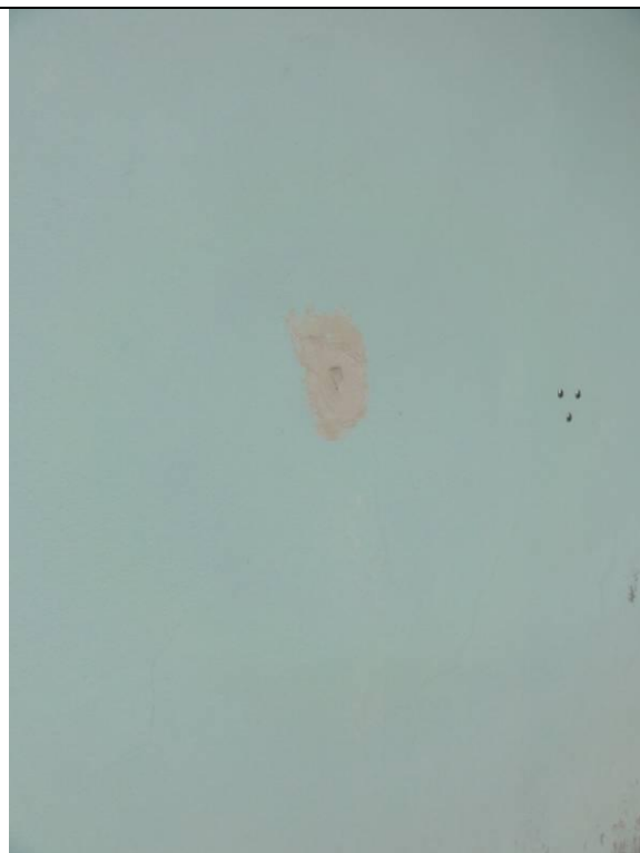
Fissura no reboco (DSC00103, 15/02/2011, 13:50h)
