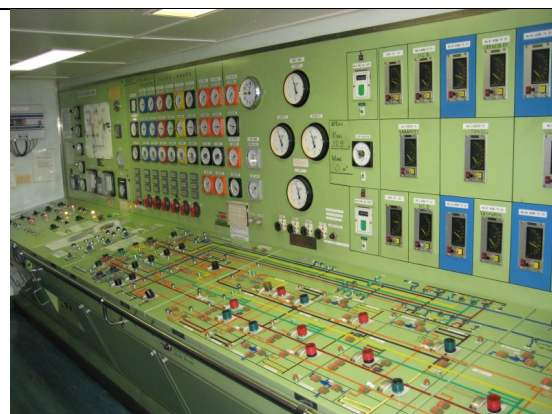
Cargo Control Room
