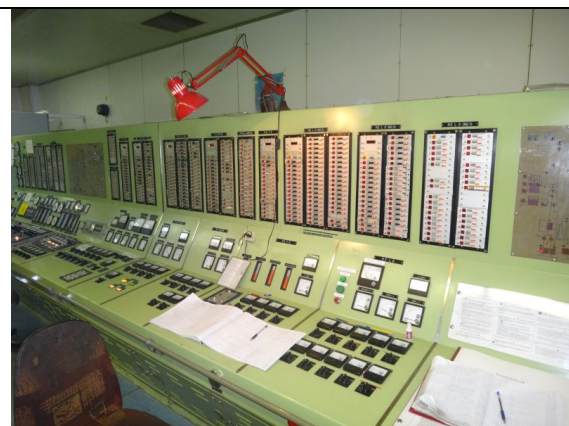
Engine control room
