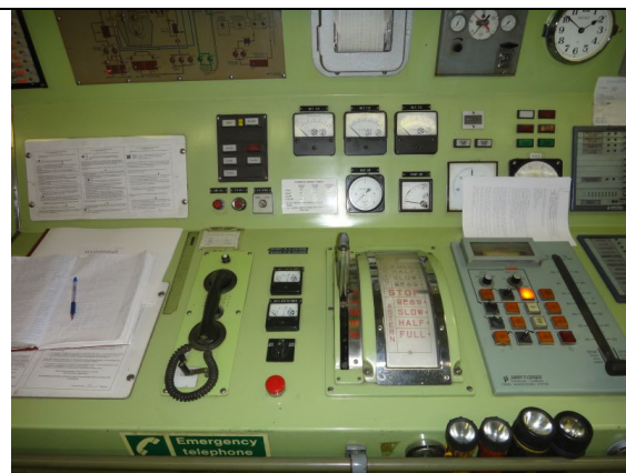
Main Engine control system
