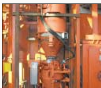
The CCB unit is the prime mover of cuttings, whether to ISO-PUMP units or directly to cuttings boxes, dryers, CRI installations or other destinations.
