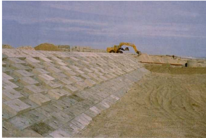
Figure 6.10 Example of emergency revetment constructed in concrete blocks, the revetment will later be buried into an artificial dune. (Danish Coastal Authority)
