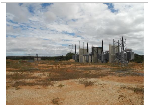
Foto 8.2.2-71 – SE Milagres II (P41, Milagres/CE). Coord. UTM 24S 508.405/9.188.394.
