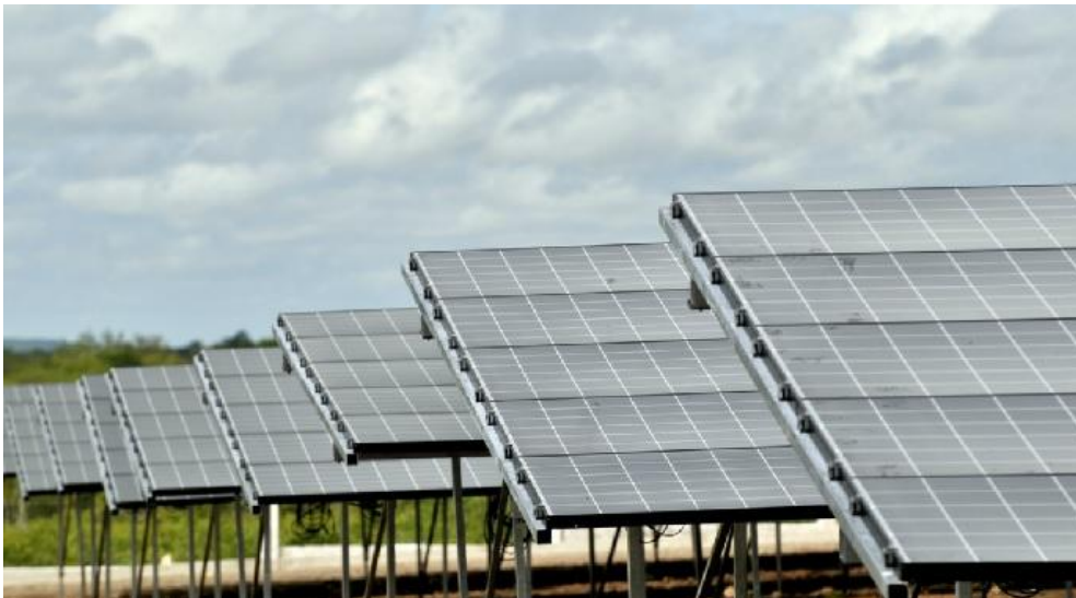
Usina Solar Tauá - CE
