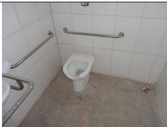
Figura 03: Reparo no PSF III
