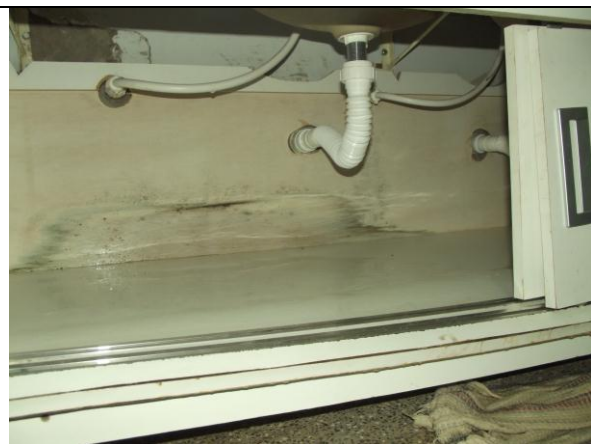
Figura 03: Reparo no PSF III
