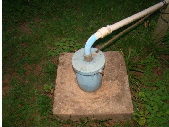
Foto 34/05 – Poço tubular profundo do Hospital Municipal.
