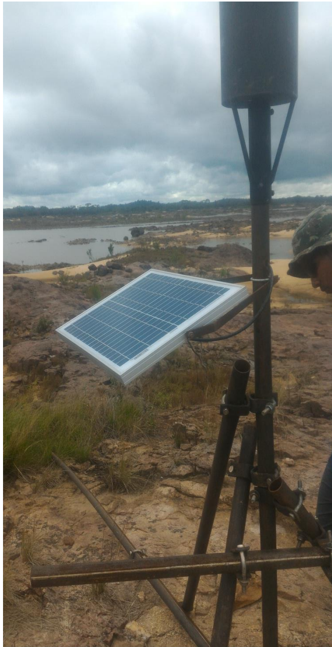
Figura 8: PCD instalada no RN03.
